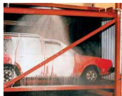
sprinkler system working
