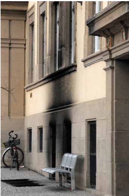
Extensive damage to the building structure. Closed 8 months for certificate (statics) and renovation.
